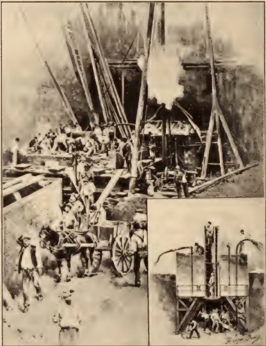
MANHATTAN LIFE INSURANCE BUILDING, NEW YORK. (Sinking the Caissons for the Foundations.)
